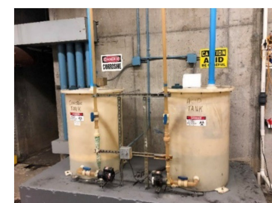
Industrial Wastewater Decontamination System
