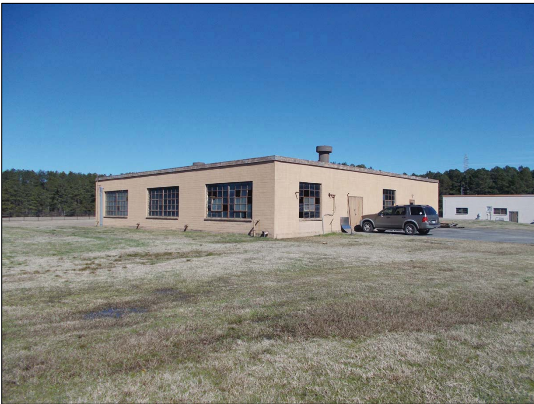
Figure 5-23. Building 20 (Cooling tower) west and south façade, view northeast; associated towers to the left and right have already been removed (DSCN1558).
