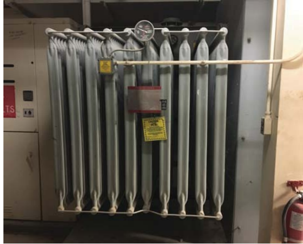
Photo 30: PCB-containing transformer in Building 53A chiller plant.
