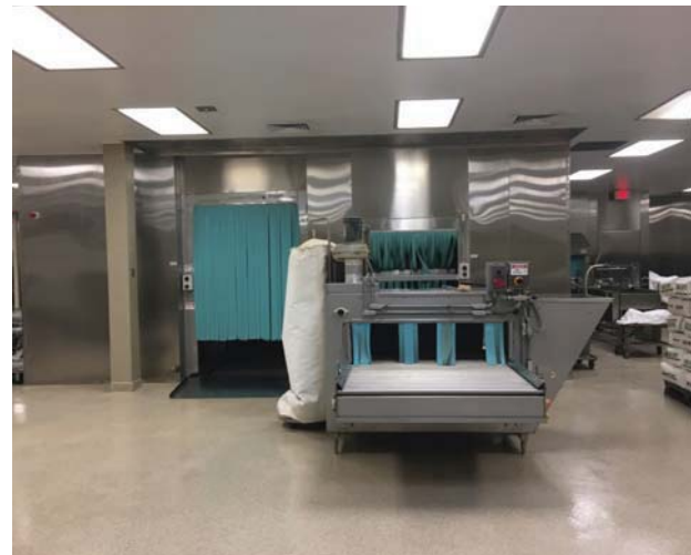
Photo 20: Processing equipment in Building 05A.
