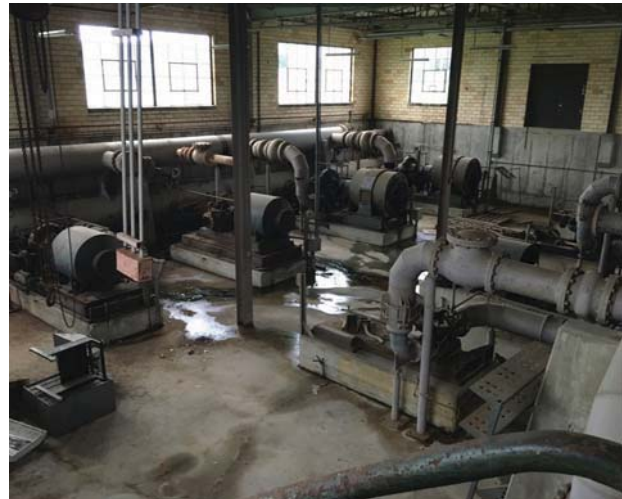
Photo 24: Out of use chiller equipment in Building 20.
