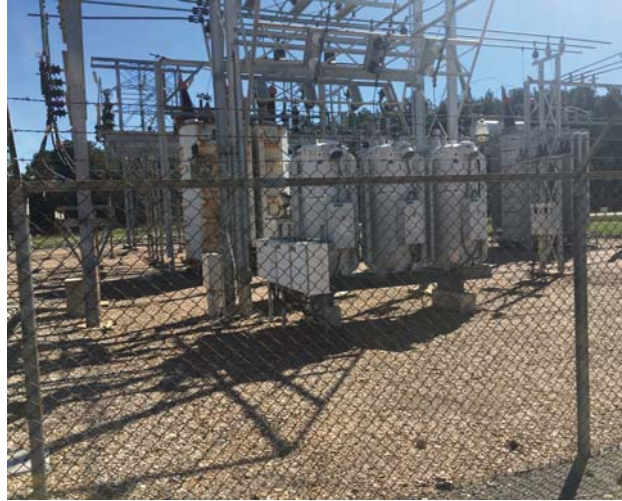
Photo 42: Transformer substation on southern portion of the Campus.
