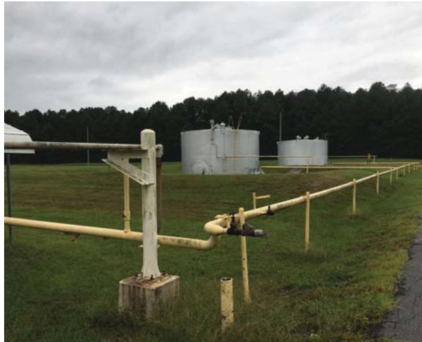
Photo 11: 28,000-gallon ASTs and piping currently in use for generator fuel oil backup.
