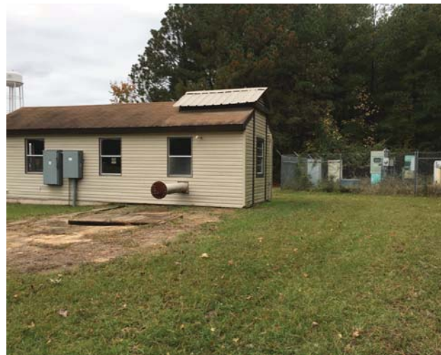
Photo 48: Well house and equipment on the north side of the Campus.
