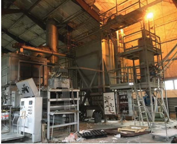
Photo 33: Building 46 incinerator (out of service) and bedding waste collection equipment.
