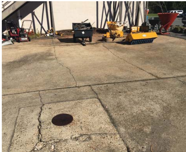
Photo 27: Concrete pad and lid (possibly indicative of a UST) south of Building 17.
