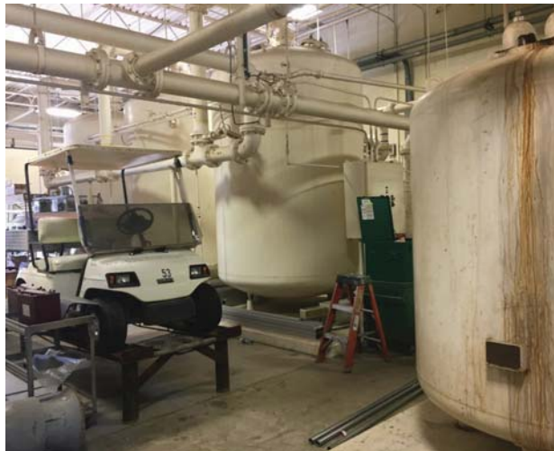
Photo 43: Former wastewater treatment tanks (no longer in operation) in Building 44.
