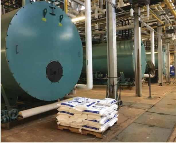
Photo 13: Boilers in Building 07.
