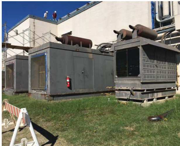
Photo 31: Emergency generators south of Building 53.
