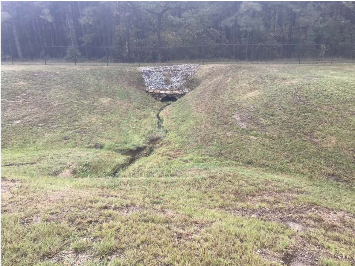
PHOTOGRAPH 10 — VIEW SOUTH OF EPHEMERAL STREAM B WHERE IT FLOWS OFFSITE. NOTE SINUOSITY AND MODERATE RIFFLE, RUN, POOL SEQUENCE.
