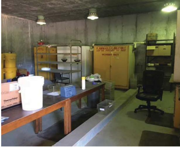
Photo 41: Hazardous waste storage in Building 37.
