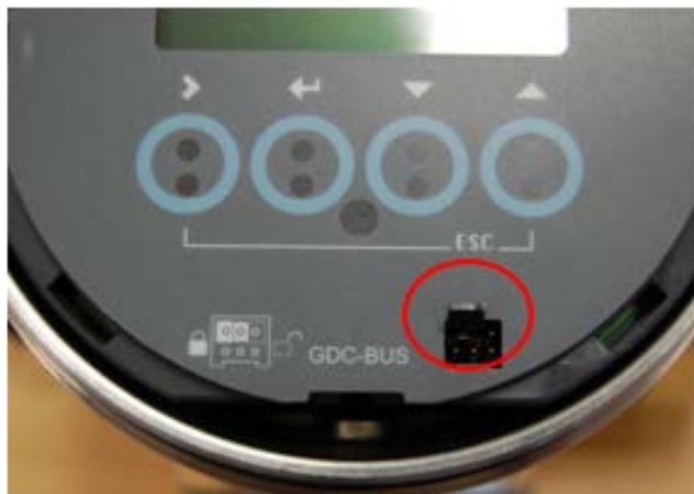
IFC300 Parameter Sealing Lock ENABLED (see 2 pins covered by protruding Tab in above photo)
